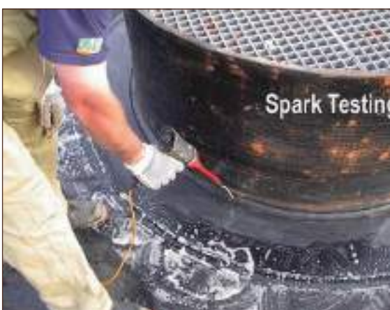
Figure A4.45 Spark testing (courtesy GSE Environmental)
